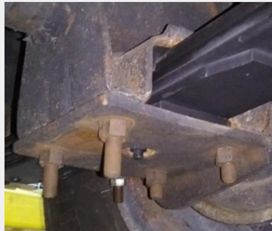
Fig 3. Leaf Spring Isolators Installed
